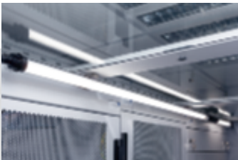
1 LED lighting → SEE P. 65
